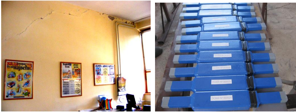
Figure 1. Typical Damages and Dampers
